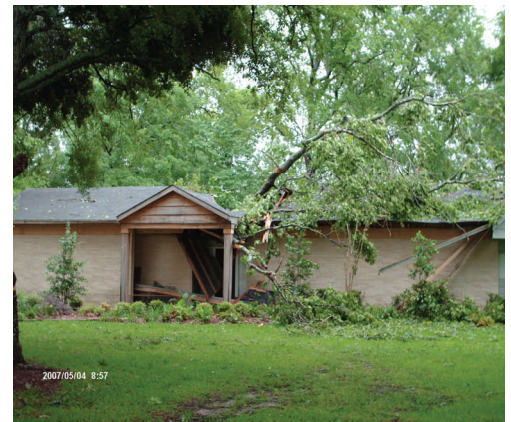
Sterlington Residence after the storm
